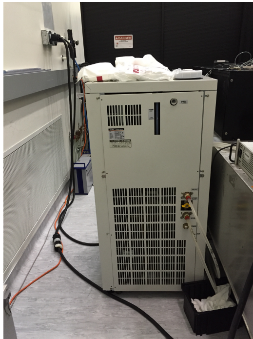
Chilled water cooler
